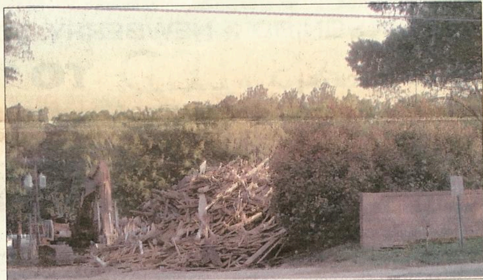
Residents have probably noticed the old jail in front of the Disabilities and Special Needs Board building being torn down the last few weeks. Here is a series of photos that shows the progression of the demolition.
